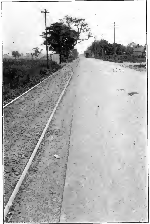
PAVING-GUARD ALONG EDGE OF A HEAVY-TRUCKING THOROUGHFARE IN SOUTH-WEST PHILADELPHIA
